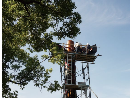
Photo 23 Temporary reinforcement of the totem pole's wings (Photo by Marie Nakamura on June 24, 2020)
